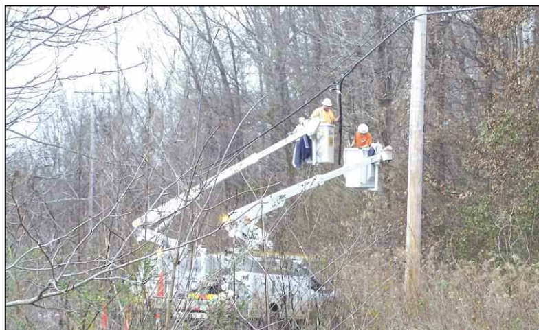
Bob Darden An AT&T repair crew works Friday afternoon to replace a section of transmission line near the Greenwood-Leflore Airport on Carroll County Road 183. Thieves took a 350- to 400-foot section of the copper cable early Friday morning.
